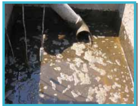
Figure 6: The sludge conditioning tank
