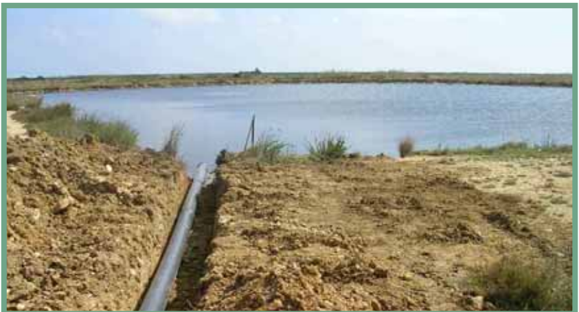
Figure 1: A large settling pond (photo STM aquatrade)
