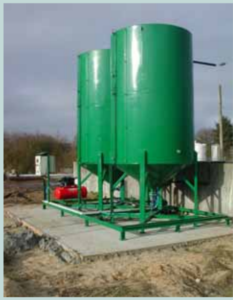
Figure 8 B: The sieve sludge sedimentation systems.
