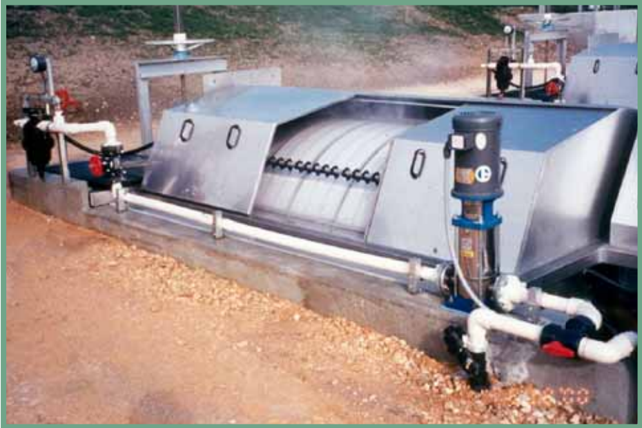
Figure 5: Drum filter (photo STM aquatrade)
