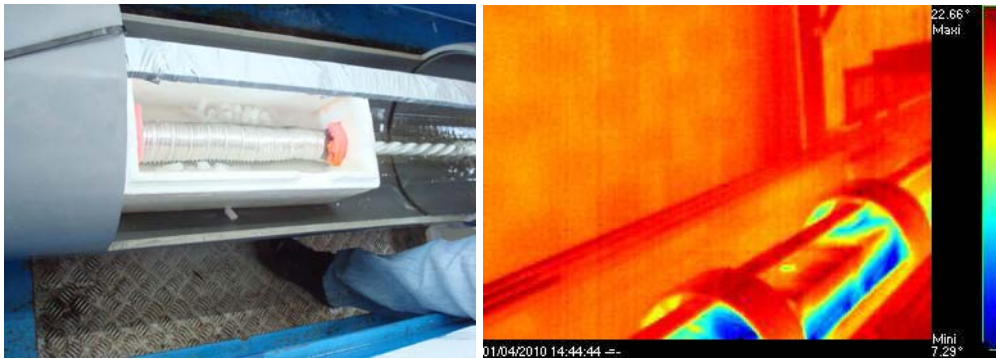
Cooling system box - IR camera image
