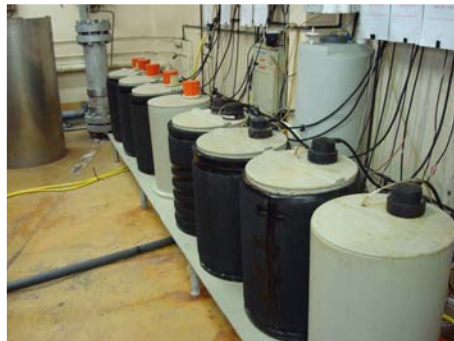
Figure 55. Circulating natural sea water tanks
