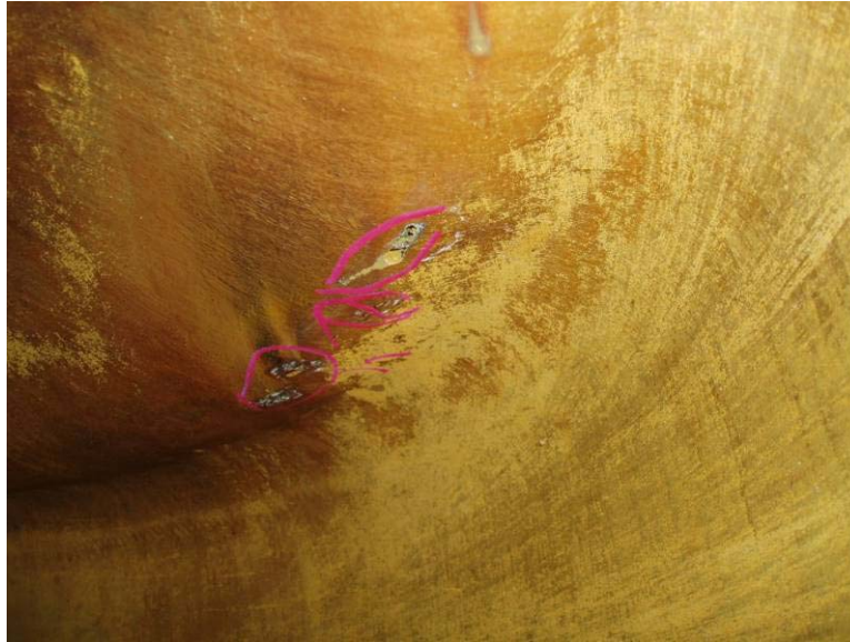
Figure 5 : Pitting corrosion of the casing of a HP booster pump (cast duplex stainless steel UNS J93550, DIN 1.4468)
