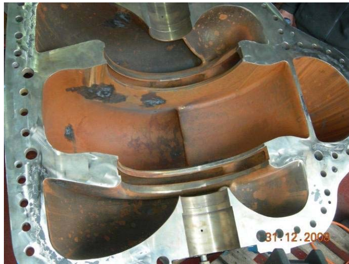
Figure 7 : Overview of the corroded pump made of cast superduplex stainless steel ASTM A890 Gr5A (UNS J93404)
