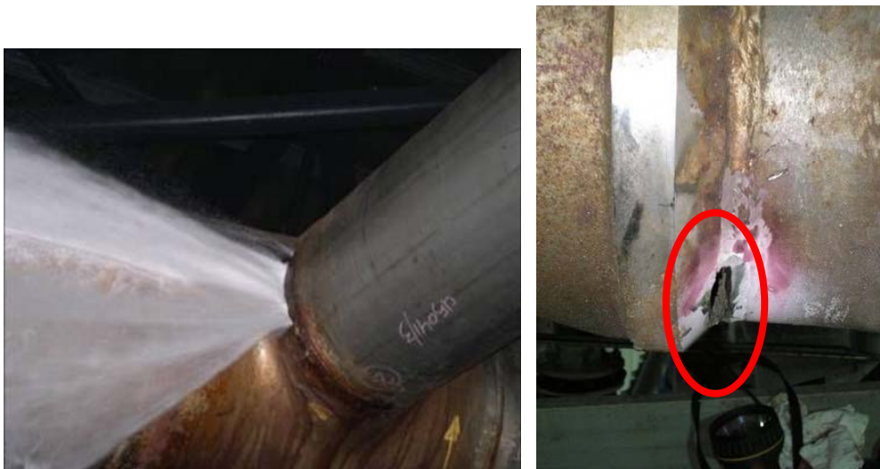
Figure 10 : Perforating pitting corrosion at welds on superduplex stainless steel pipes. In these cases, welding was not performed according good engineering practices.
