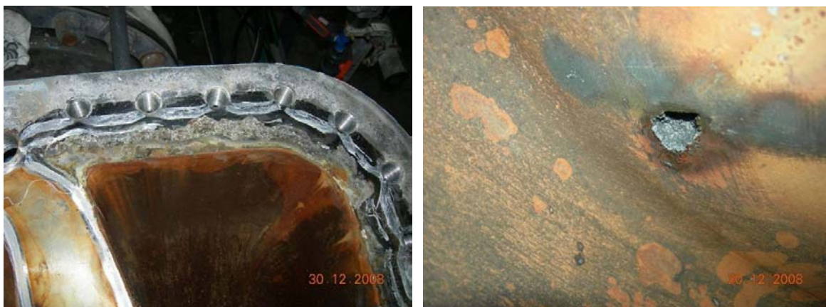
Figure 8 : Crevice (a) and pitting (b) corrosion of pump made of cast super duplex stainless steel ASTM A890 Gr5A (UNS J93404)
