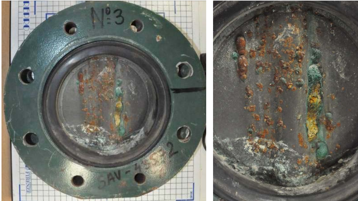
Figure 11 : Aspect of the corroded valve
