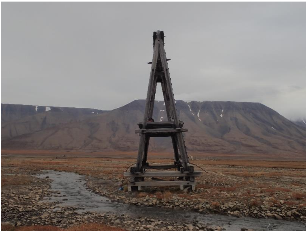
Figure S1.f. Uneven settlement (tilt to the left) of the cable post Nr. 10 at Line 6 (05.09.2021, location f in Table S1), Adventdalen. It is suggested that the settlement occurred due to stronger degradation of permafrost due to warming effect of small river running next to it. Photo: © Anatoly Sinitsyn/Sintef.
