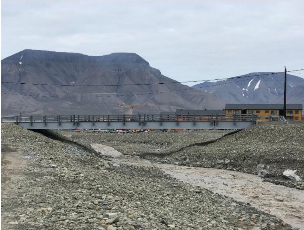
Figure S1.a10-3. Longyearelva running through engineered riverbed below the bridge over the Road 501 (17.08.2021). Photo: © Anatoly Sinitsyn/Sintef.
