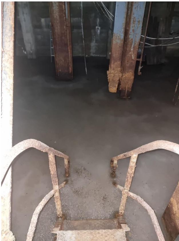
Figure S1.l. Stairs and ground floor at Gamle kraftstasjonen (The Old Power Plant) in Ny-Ålesund, which is permanently filled with ice (12.07.2023, location l in Table S1). Photo: © Ingrid Rekkavik/Kings Bay AS.
