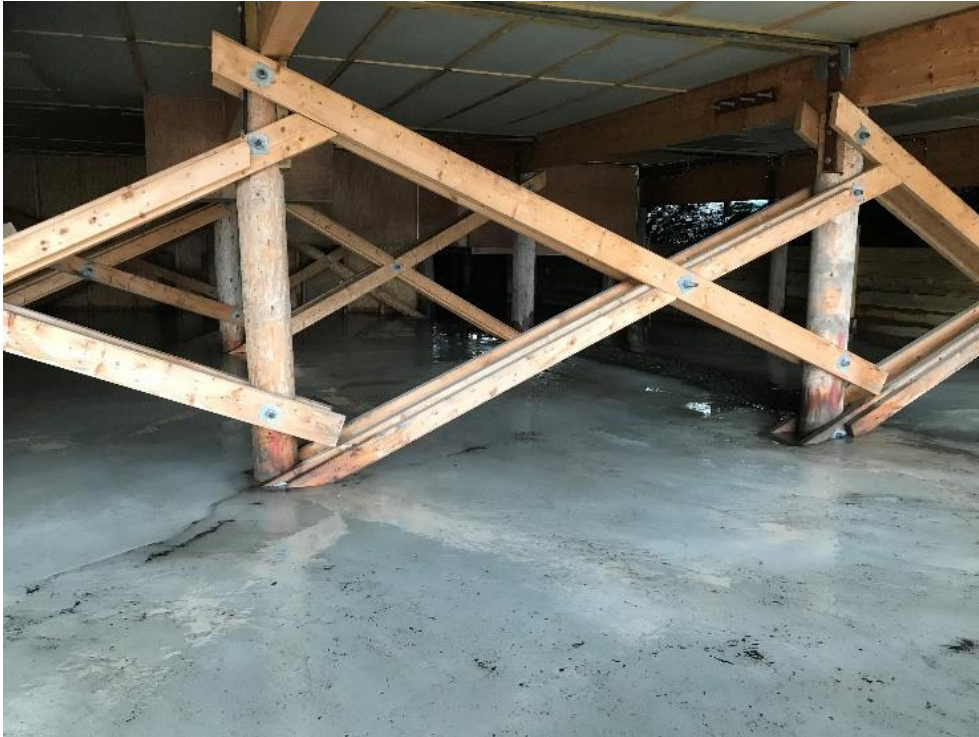
Figure S1.a3. Medium-size, "flat and spread" not cracked icing at location under the building Nr.1 and the Road 509, Elvesletta Nord (18.06.2017, location a3 in Table S1). Photo: © Anatoly Sinitsyn.
