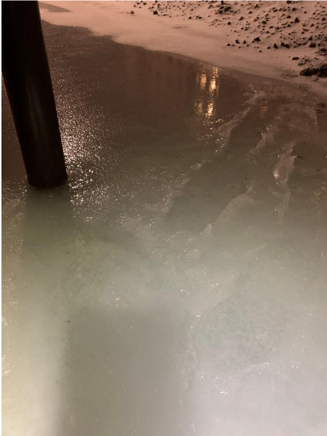
Figure S1.a11-1. Icing below housing for student's accommodation in Elvesletta (09.11.2021, location a11 in Table 1). Photo: © Tove Trondsen/Norges arktiske studentsamskipnad.
