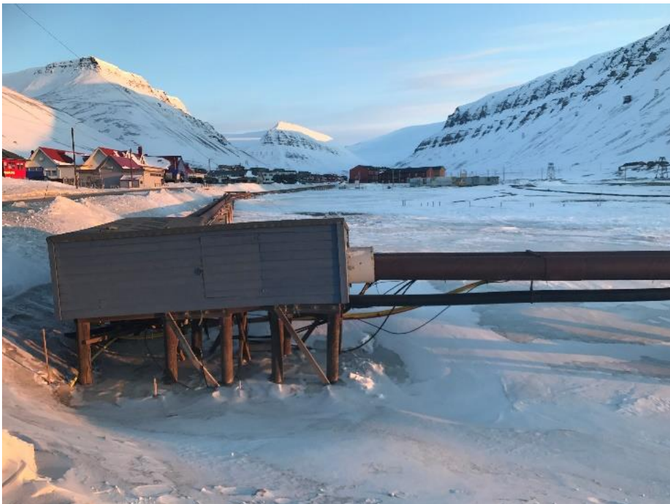
Figure S1.a4. Medium-size, not cracked icing at Elvesletta affecting supporting structure for pipeline on its turning point (18.04.2017, location a4 in Table S1). Photo: © Anatoly Sinitsyn.
