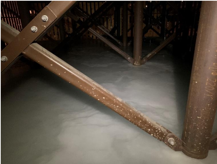
Figure S1.a11-2. Icing below housing for student's accommodation in Elvesletta (09.11.2021, location a8 in Table 1). Photo: © Tove Trondsen/Norges arktiske studentsamskipnad.
