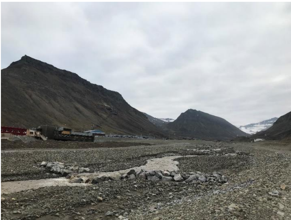
Figure S1.a10-4. Longyearelva running through engineered riverbed above the bridge over the Road 501 (17.08.2021). Photo: © Anatoly Sinitsyn/Sintef.
