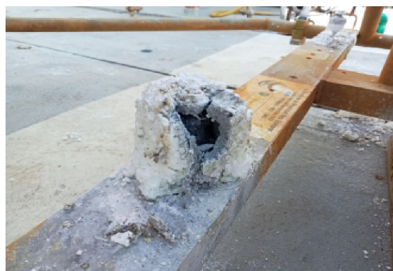
Figure 32 : Photo de corrosion
