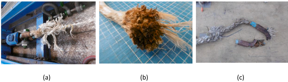
Fig. 8. Failure zones, a) at end of splice, example I-2, b) damaged strand due to thimble, sample I- 7, one of three severed strands, c) broken steel thimble, I-9.
